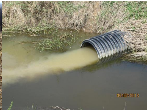
Sediment exiting tile, likely originating from surface riser.
